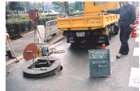
Lifting the machine with a crane after the completion of cutting work
