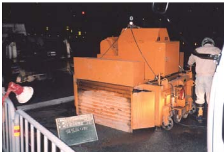
A shutter provided to enclose the machine during cutting work for preventing concrete pieces from flying and reducing noise level.
